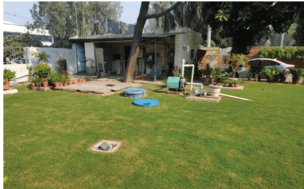
Two underground RWH units with two lakhs litres storage capacity
