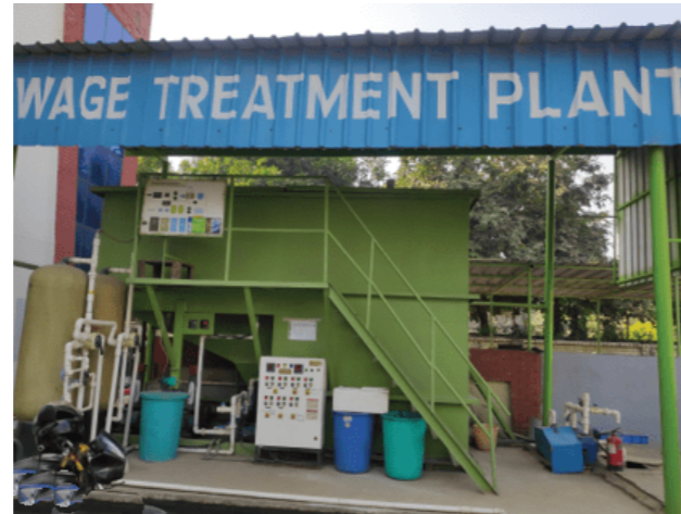
Sewage Treatment Plant
