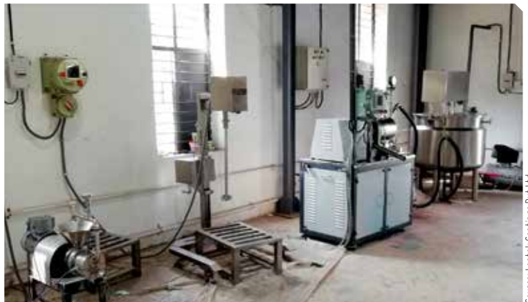
Shop floor and machinery at Leotek Coatings Pvt Ltd
